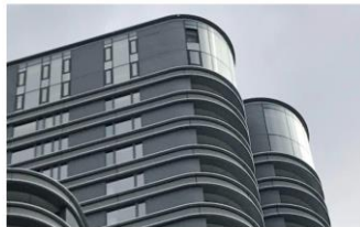
A window is seen to be missing from the 27th floor of the building. ©BBC/PA
