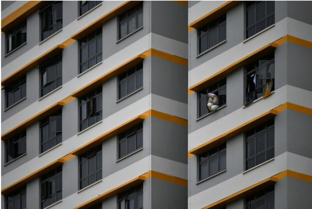
Homeowners can prevent falling windows by checking and maintaining their windows at least once every six months, said BCA. ST PHOTO: LIM YAOHUI
