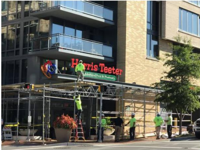
Workers install protective scaffolding over the entrance to a building at 8300 Wisconsin Ave. in Bethesda on Aug. 30, 2019, a week after a glass railing shattered and fell to the sidewalk from a ninth-floor balcony, injuring a 12-year-old girl. (Katherine Shaver/The Washington Post)
