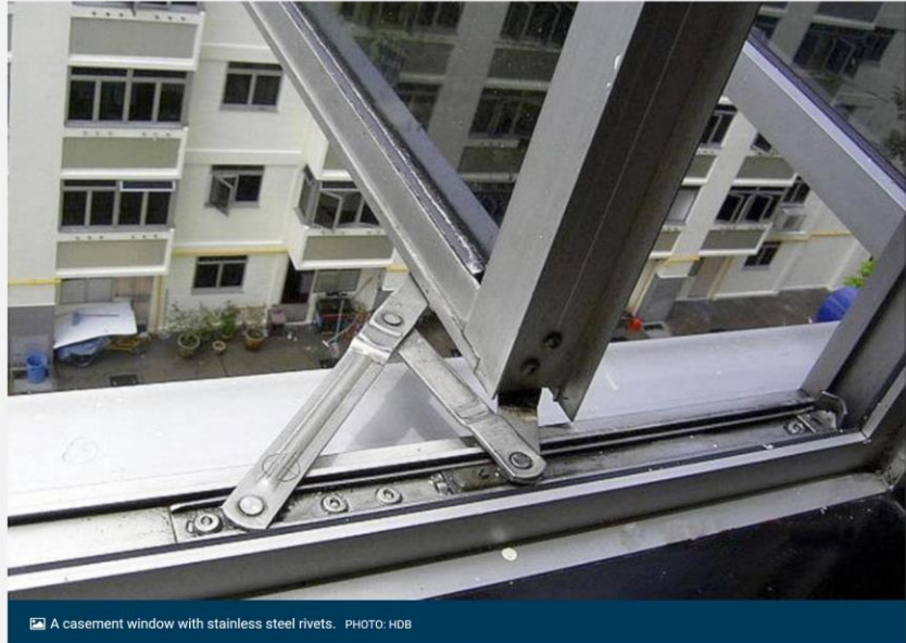
A casement window with stainless steel rivets. PHOTO: HDB
