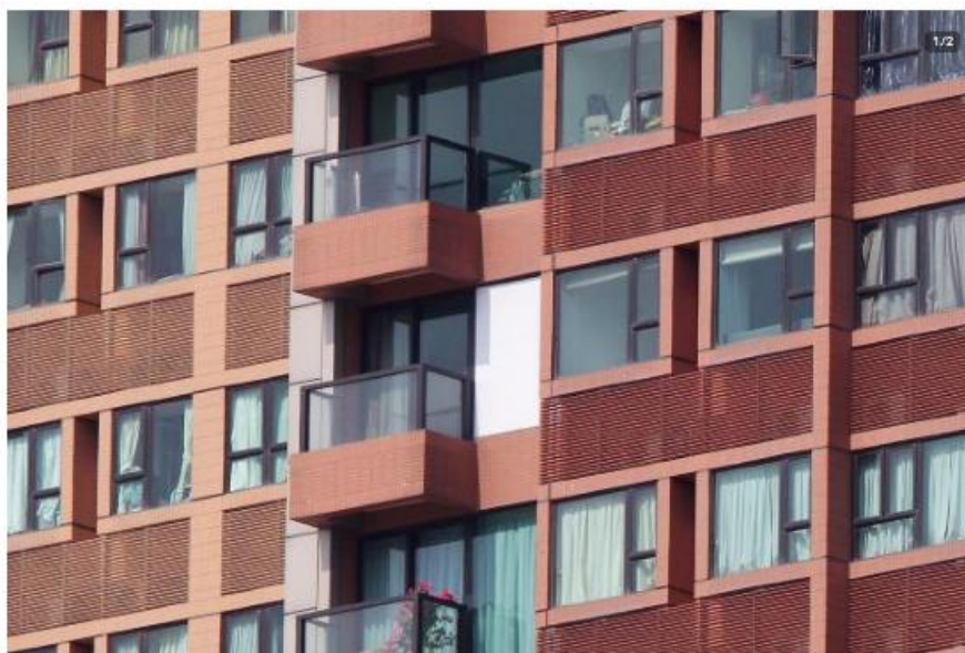
A white cover masks a broken window at The Arch in West Kowloon. Residents fear the breakages will reduce the value of their flats. Photo: Felix Wong
