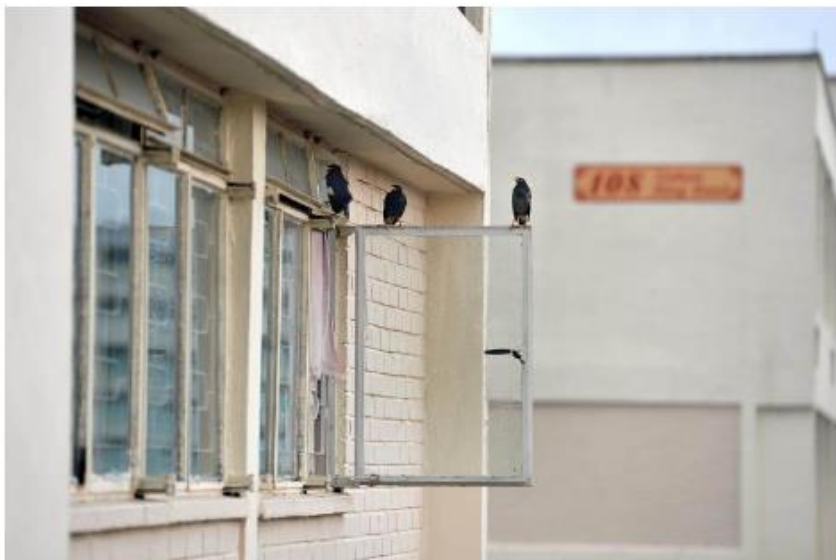
There have been 50 cases of windows falling this year, with the Building and Construction Authority (BCA) and the Housing Board (HDB) reminding home owners to maintain their windows at least once every six months. PHOTO: THE NEW PAPER
