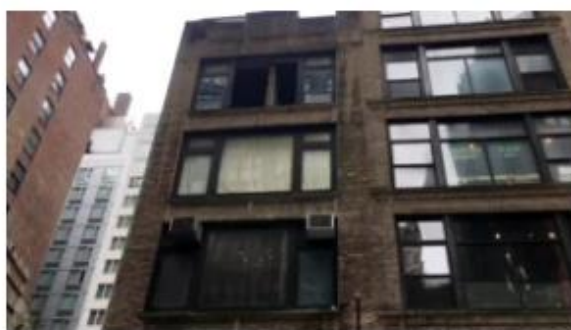
A pane of glass fell from a building on 38th Street in Midtown on Sept. 13, 2018. (credit: Dave Carlin/CBS2)
